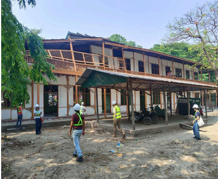
Photo: UNOPS engineers conduct a Rapid Damage Assessment of a basic education middle school near the epicentre.
